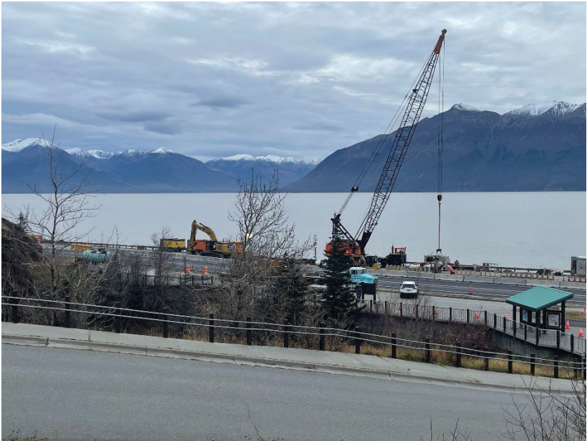
Photo 24: Looking south at construction activities on the railroad tracks along the Cook Inlet side of the highway near Mile 112 of the XSC. (November 2, 2023)
