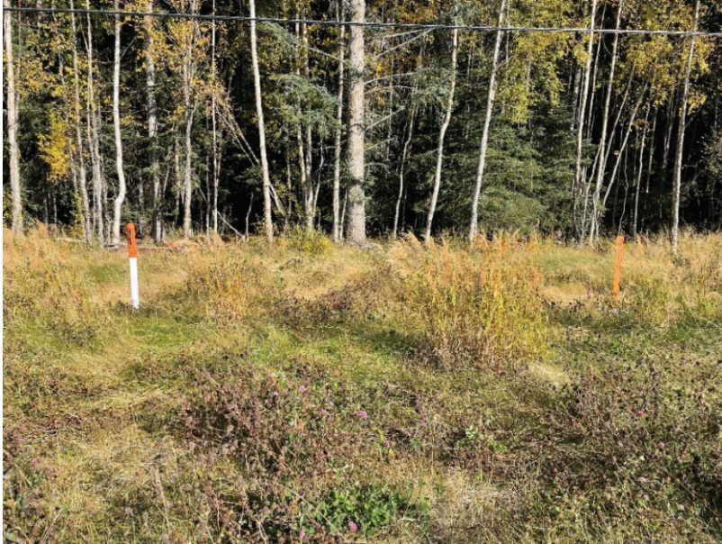
Photo 5: Looking northeast at buried a buried fiber optic cable along the Seward Highway near Mile 100.5 of XSC. (September 27, 2023)
