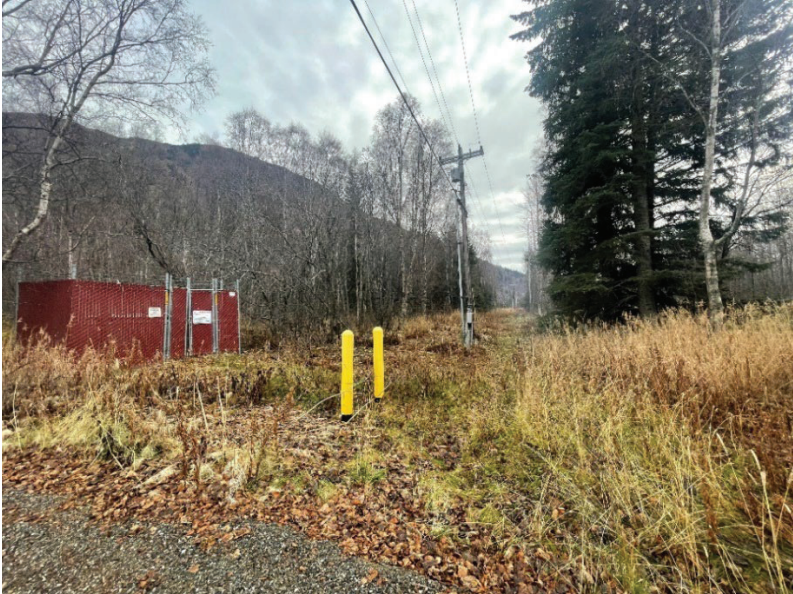
Photo 13: Looking south at powerlines and CEA pole-mounted transformer, buried natural gas pipeline markers, and fenced-in ENSTAR pipeline access, located east of the Valley Bible Chalet. (November 2, 2023)
