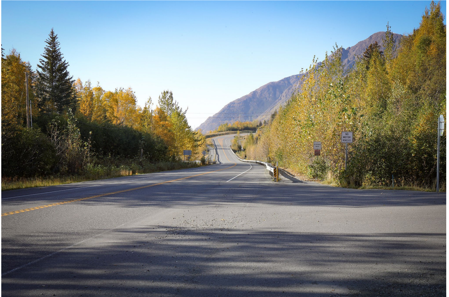
Figure A-13. Existing view of Bird Creek Bridge, from approximately MP 101.25, facing north.
